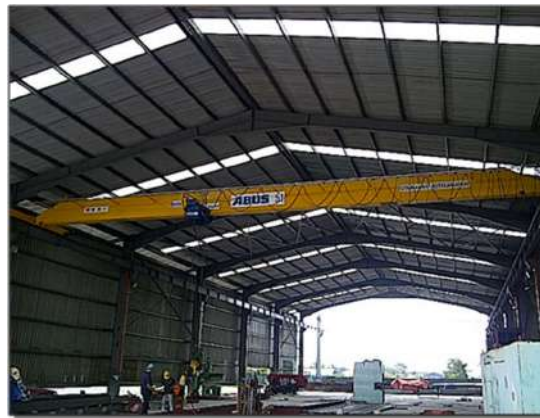
OVERHEAD CRANE 5 ~ 50 TONS
