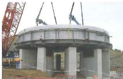
Koniambo Furnace Bottom Support Ring and Water-cooled Hold Down Ring Beam Total Mass: 270 000 Kg
