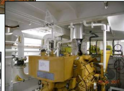
Auxiliary engine room
